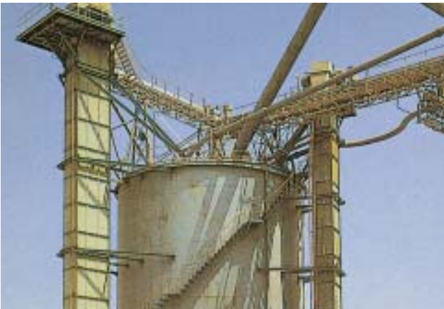
Bucket elevator (NE type)
